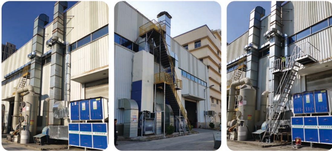
Three sets of painting and spraying waste gas treatment equipment added by Shenzhen plant during the reporting period
