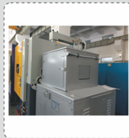
Furnace safety guard
